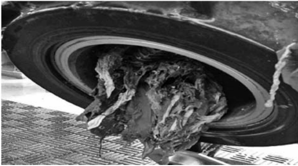
Photo. 7 Foreign Substances Clogged in the Pump
