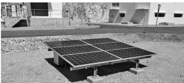
Photo. 4 Electric Power Generation by Solar Panel
