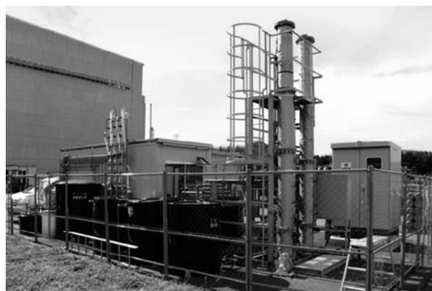
Photo 1 Pilot-scale SWRO plant in Tokyo Bay
