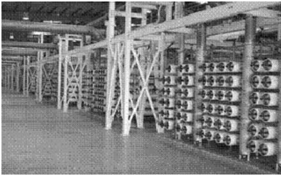
Fig. 3 The world's largest municipal wastewater recycling plant (Kuwait)
