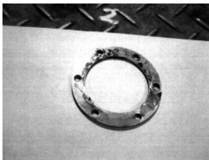
Photo. 2 The metal weight ring corrosion situation
