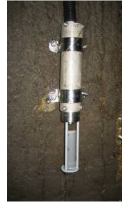
Photo.2: Installation situation of the water level sensor
