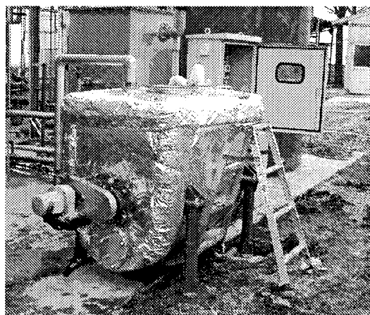
Fig.2 Externals photograph of test fixture
