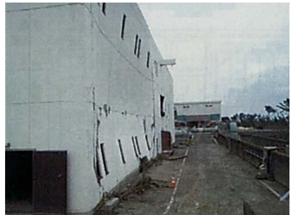
Photo. 4. 4 Wall of the main pump building. Tsunami came and struck the building from the right side in the photo and bent the wall
