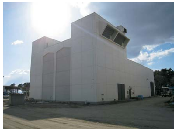
Photo. 4.7 Housing of the emergency generator facility (Photograph taken in Apr.2011) Major damage could not be seen on this building.
