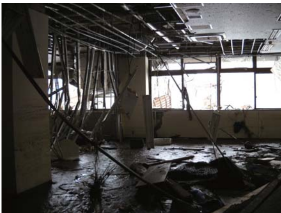
Photo. 2.3 Interior of the administration building on the 1st floor (Photo taken by staff member at the STP in Mar., 2011)
