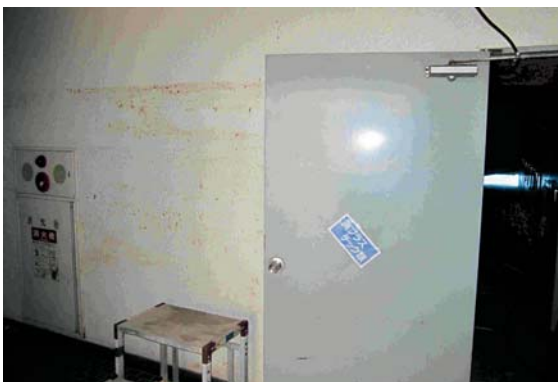
Photo. 3.9 Tsunami trace on the electrical room entrance on the 1st floor of the sludge treatment building (Photo taken in Nov. 2011)
