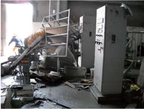
Photo. 2.7 Local control panel of the sewage pump on the 1st floor (Photo taken by staff member at the STP in Mar. 2011)
