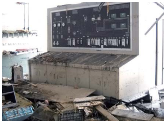
Photo. 2.11 Submerged sludge-treatment monitoring room on the 1st floor (Photo taken by staff member at the STP in Mar. 2011) Inundated up to ceiling level by the Tsunami
