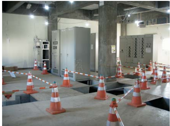
Photo. 5.5 Restoration status of local electrical room (Photo taken in Dec. 2011)
