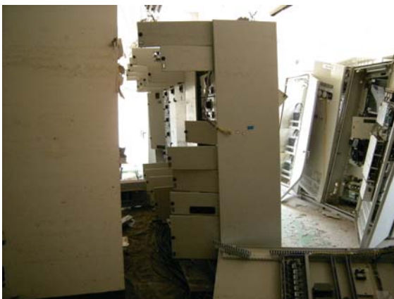
Photo. 5.3 Damaged electrical room (Photo taken in Apr. 2011) Electrical equipment was inundated or destroyed by the Tsunami
