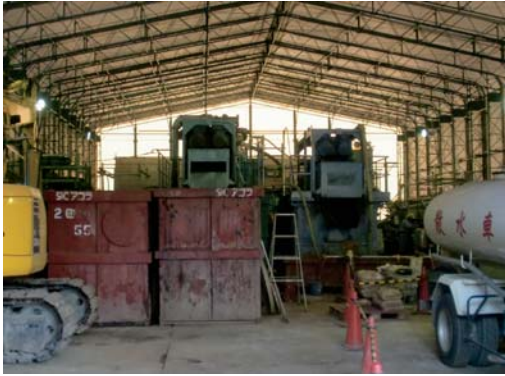
Photo. 3.7 The temporary dehydrator (Photo taken in Nov. 2011) Sludge brought about by the tsunami is treated using the temporary dehydrator.
