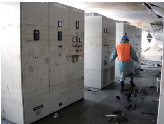
Photo. 2.10 Electrical room in the dehydrator building area (Photo taken by staff member at the STP in Mar. 2011) Inundated because it was installed on the 1st floor
