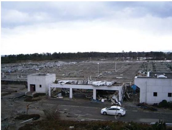
Photo. 5.2 The destroyed upper part of the water treatment facilities (Photo taken in Apr. 2011)
