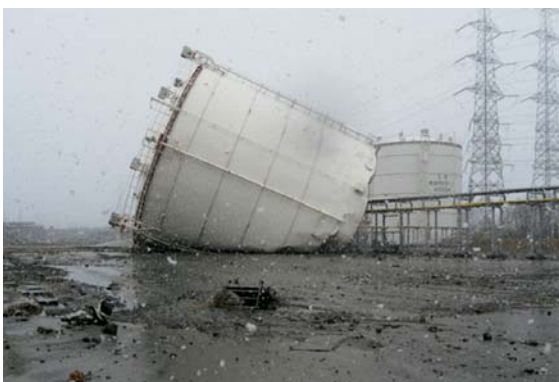
Photo. 3.3 Toppled digestion gas tank (Photo taken by staff member at the STP in Mar. 2011)
