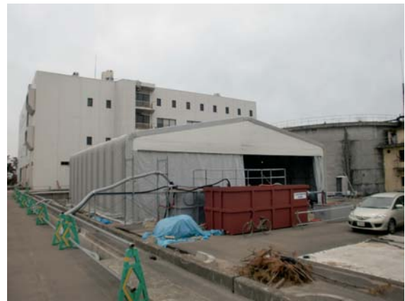
Photo. 4.13 Temporary dehydrator housing. (Photograph taken in May 2011)
