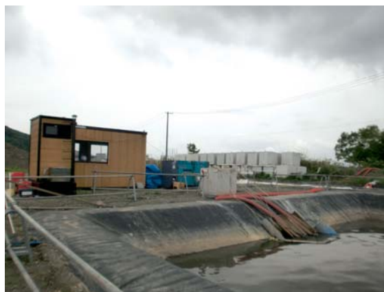
Photo. 2 A temporary sedimentation pond and discharge pump was installed near the watershed of the Kyuukitakamigawa River to treat sewage water right after the earthquake. (Date Taken : May 2011 at near Ishinomaki Tobu STP)
