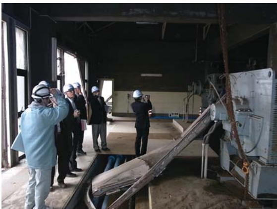
Photo. 1.1 Survey conducted at the emergency generator room in Ken-nan STP (Photo taken in Nov. 2011)
