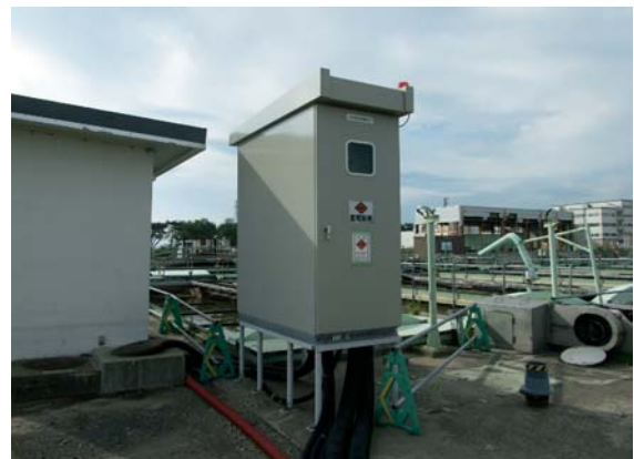
Photo. 4.8 Temporary receiving power unit 6.6 kV installed on the primary sedimentation tank. (Photograph taken in May 2011)
