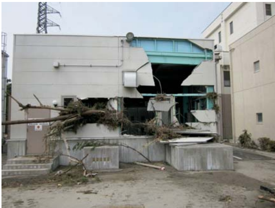
Photo. 4.6 Housing for the high voltage power Largely damaged wall because of drift wood.
