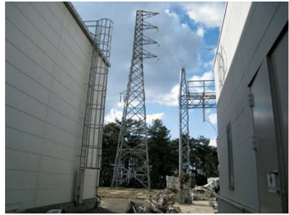
Photo. 4. 3 Electrical towers. (Photograph taken in April 2011) The electrical tower withstood the Tsunami attack. It did not collapse and was not damaged.
