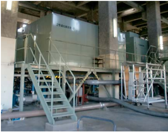
Photo. 3.13 Centrifugal dehydrator installed on the high frame (Photo taken in Nov. 2011) Not inundated because installed at elevation, but auxiliary equipments were broken
