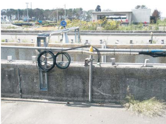
Photo. 4.10 Temporary inflow meter (Photograph taken in April 2011) It is installed temporarily at the inlet of the STP.
