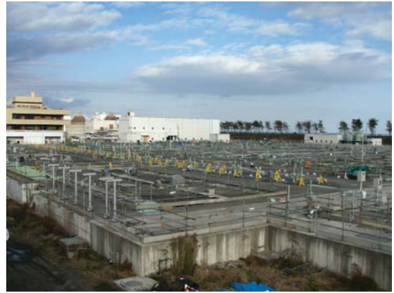
Photo. 5.4 Restoration status of destroyed upper part of water treatment facilities (Photo taken in Dec. 2011)
