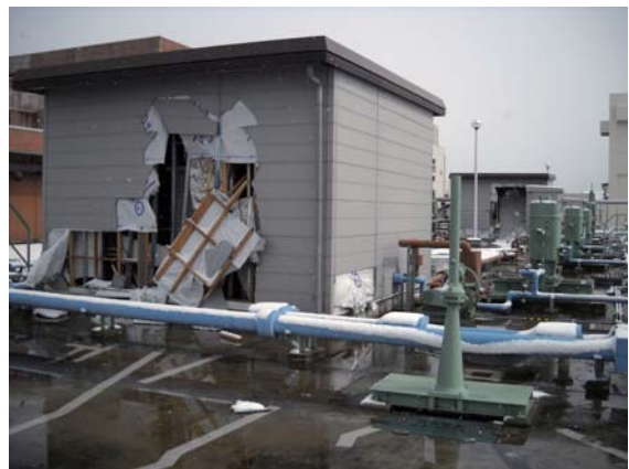
Photo. 2.6 Upper part of the outdoor biological reactor tank on the 2nd floor of the building (Photo taken by staff member at the sewage treatment plant in Mar. 2011)
