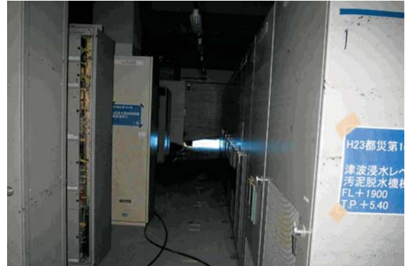
Photo. 3.10 Tsunami trace in the electrical room on the 1st floor of the sludge treatment building (Photo taken in Nov. 2011)
