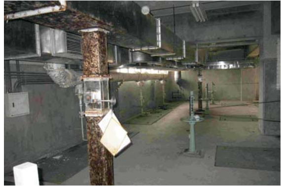
Photo. 2.4 Upper part of the indoor biological reactor tank on the 2nd floor (Photo taken in Nov. 2011) No significant damage to the building structure was found.
