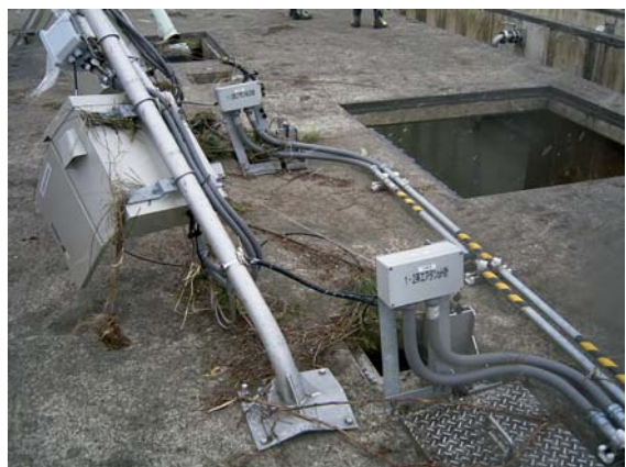
Photo. 5.6 The destroyed pH meters for Aeration Tank No. 1 and 2 (Photo taken in Apr. 2011) Mounting pole destroyed by the Tsunami
