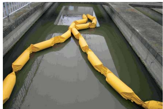
Photo. 3.12 The disinfection tank (Photo taken in Nov. 2011) Disinfection was performed strictly for sanitation.
