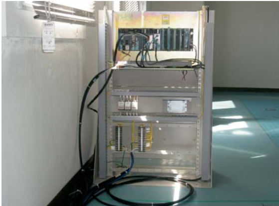
Photo. 4.9 Temporary sludge treatment controller (Photograph taken in May 2011) It is installed in the electric room on the 4 th floor of sludge treatment building.
