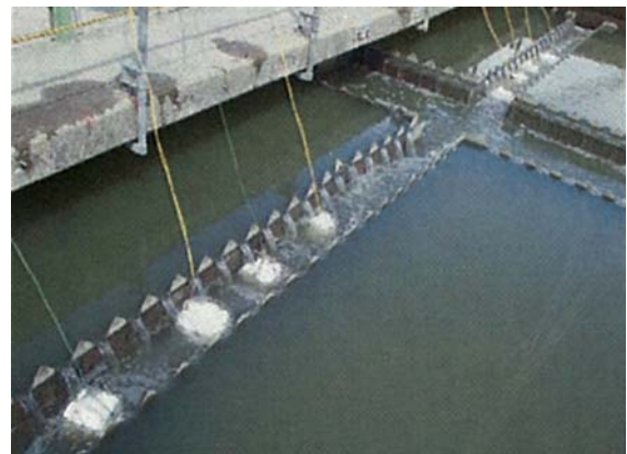
Photo. 4.11 Disinfection with solid chlorine
