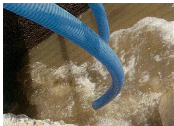
Photo. 4.12 Injection of hypochlorous acid in temporary facility
