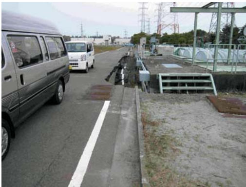
Photo. 3.8 Caved-in road within the facilities because of ground liquefaction (Photo taken in Nov. 2011)
