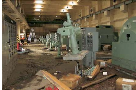
Photo. 3.4 Damaged blower equipment (Photo taken by staff member at the STP in Mar. 2011)
